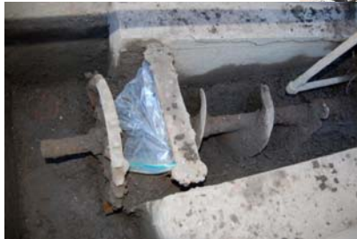
Unit 2 inside the main dye works, the grain screw conveyor and underground trough
